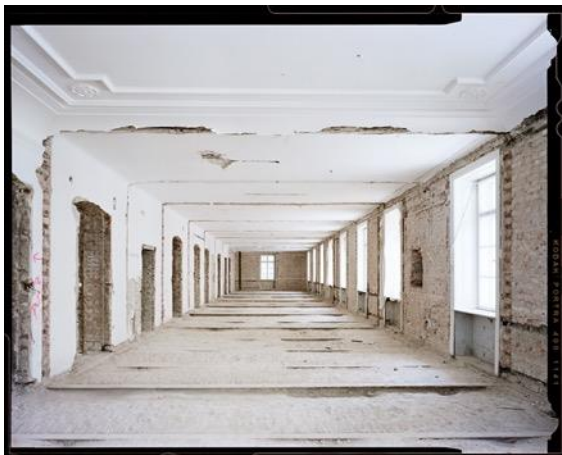
Documentation of the construction site, Photo: Stefan Oláh, © Heidi Horten Collection, Bildrecht Vienna, 2022
